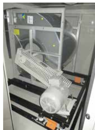
Figure 5: Belt Driven Fans & Motors
